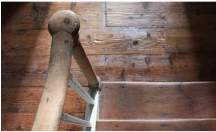
Timber handrail softened by time
